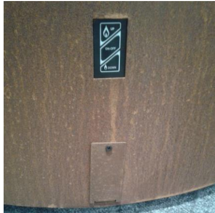
Photo 5: Receiver batteries containers
